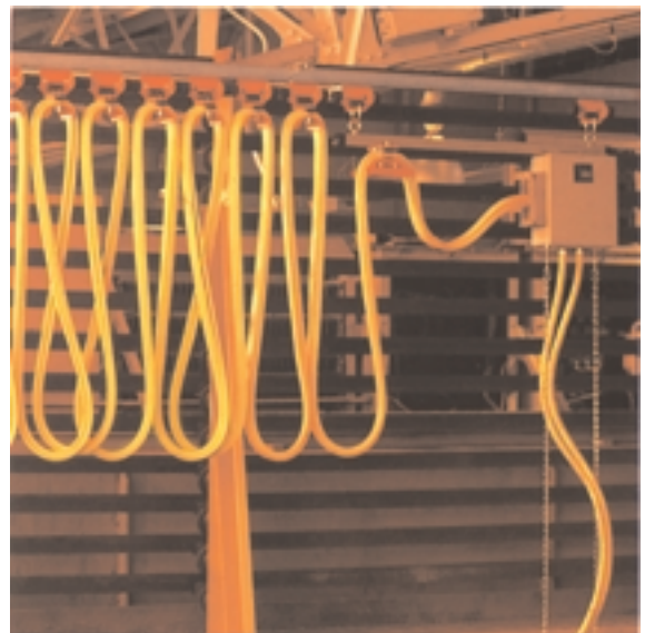
ON THE COVER: Typical Gleason C-Rail festoon system providing traveling pendant control to an overhead crane.
